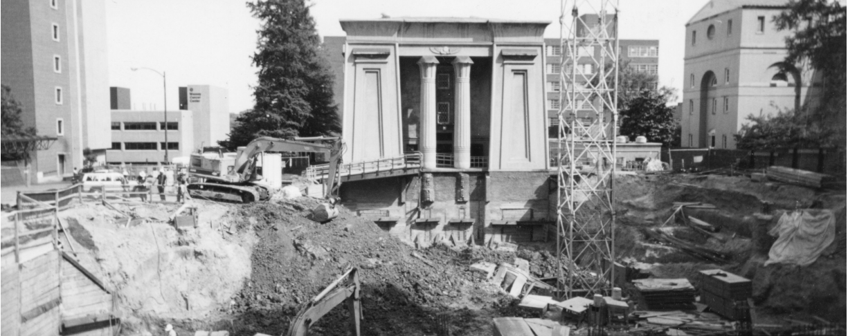
The original foundation of the Egyptian Building was laid bare during construction of a new medical sciences building in 1994.
