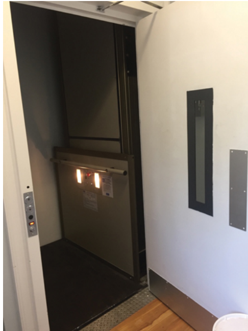
Figure 21-3 Vertical platform elevator for wheelchair users.
