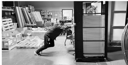
James pushing a server rack
